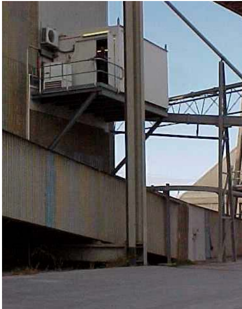
Figure 1 A Continuous On-Stream XRD Analyser installed at the finish mill.
